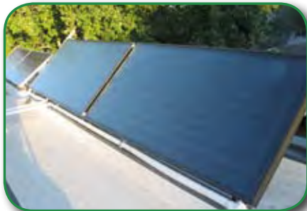
Solar Hot Water Panels.
