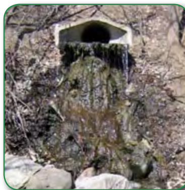
Pipe outfall discharging into the Mississippi/Minnesota confluence, just south of the Hiawatha Corridor.
