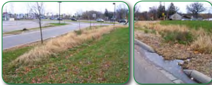
Linear infiltration area with curb cuts to allow drainage from the transit lot area.
