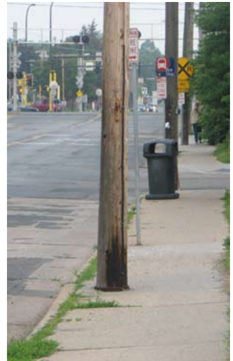
Above photo shows the poor condition of 38th Street, particularly for pedestrians, bicyclists, and transit riders.
